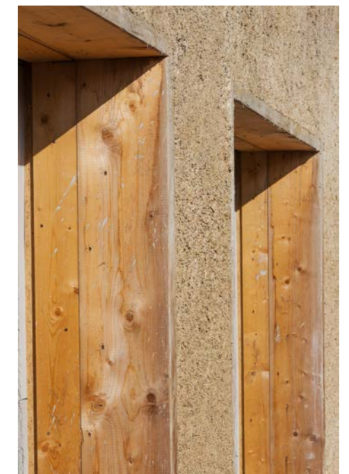
Image of low carbon wall build-up: hemp & lime insulating material within timber-framed facade
