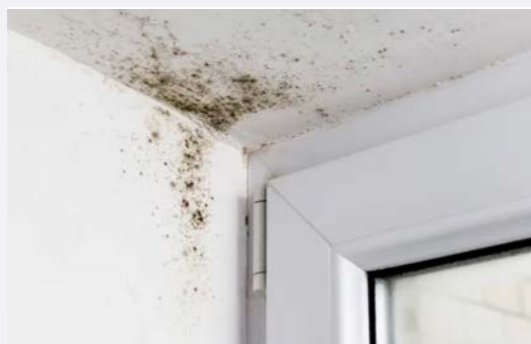
example of mould growth at window resulting from poor ventilation
